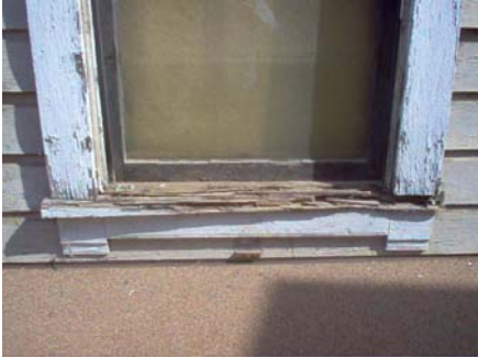
Termite Damaged Sill on the South Elevation
