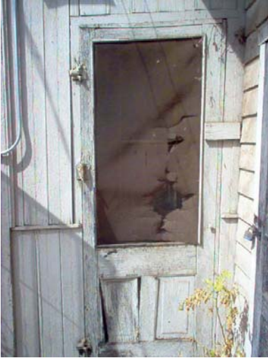
Heavily Damaged Exterior Door on East Elevation
