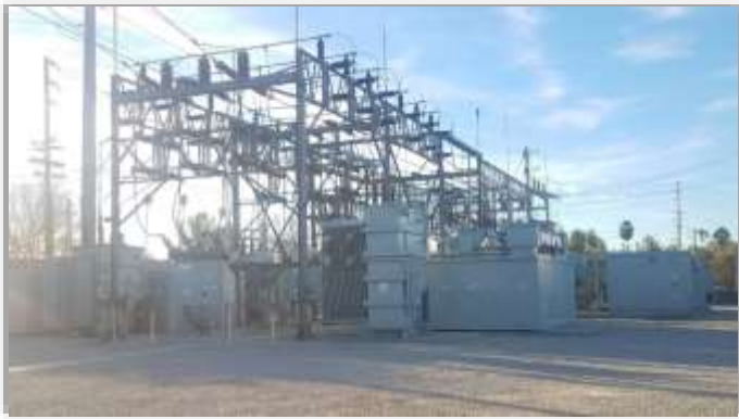
Existing Hunter Substation
